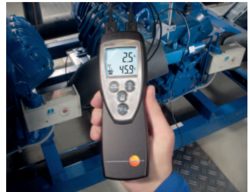
Simultaneous measurement of overheating and undercooling in refrigeration plants with testo
